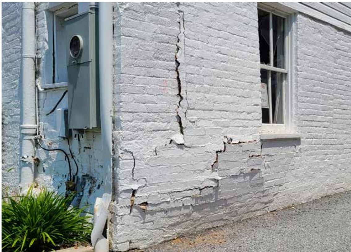
The initial impact was on the rear wall but the stress rippled through the structure to damage the east wall.
