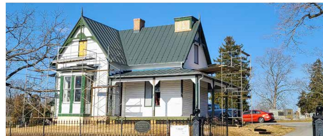
The Elmwood Cemetery Association has begun long-needed repairs to the roof, gutters, windows and siding of the caretaker's house on Kearneysville Pike, just south of Shepherdstown. The association plans to restore the interior next.
