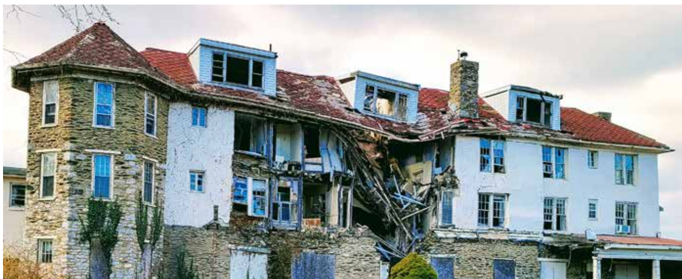
A last look at the current Hill Top House in Harpers Ferry before construction work began in late January 2022. Swan Hill Top, the development company, says that the activity of the early stages of the project may not be very visible as workers clean up and deconstruct the interior of the building to salvage wood, stone, and other materials for reuse in the new structure.
