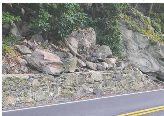
The unstable rock above this stretch of road poses a persistent danger along this heavily-traveled route.
