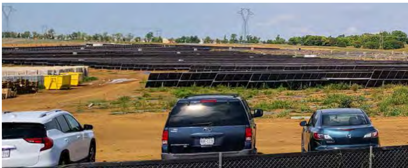
The Blake industrial solar facility appears to be employing a lot of workers for the construction on its 500-acre site in Kabletown. Looking at the cars in the temporary parking lot, you can see lots of license plates from Texas, Florida, and other far-flung states but very few from West Virginia.
