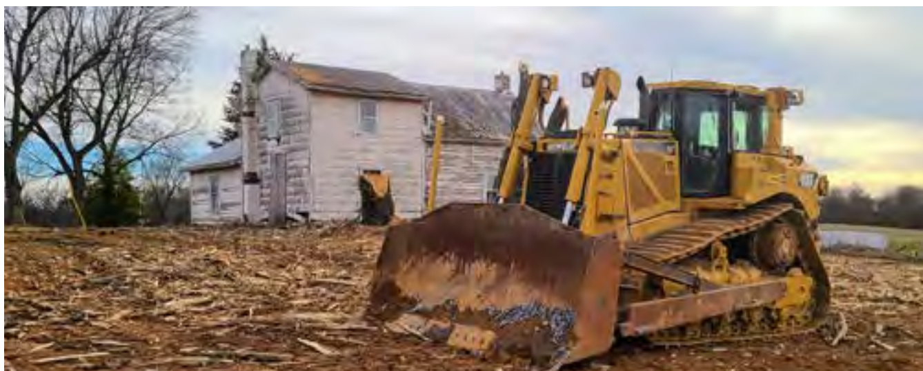
West Virginia's Division of Highways has started work to widen Route 340 to the south of Charles Town. The project will connect the existing two-lane section of the road to a new two-lane roadway that will pass to the east of the historic Rippon village (behind the post office) then cross back over and run west of the existing single-lane roadway to avoid the historic Shady Grove Farm that straddles the border with Virginia. The path of the new road runs directly through the front door of the Rainbow Road Club, where singer Patsy Cline performed in the 1950s (story, page 7).
